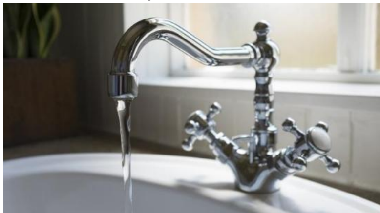
Figure 6.10: A Typical examples of Pipe borne water inside Dwelling
